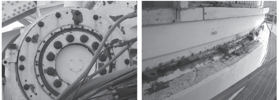
Figure 2: External corrosion on 70-meter antenna
