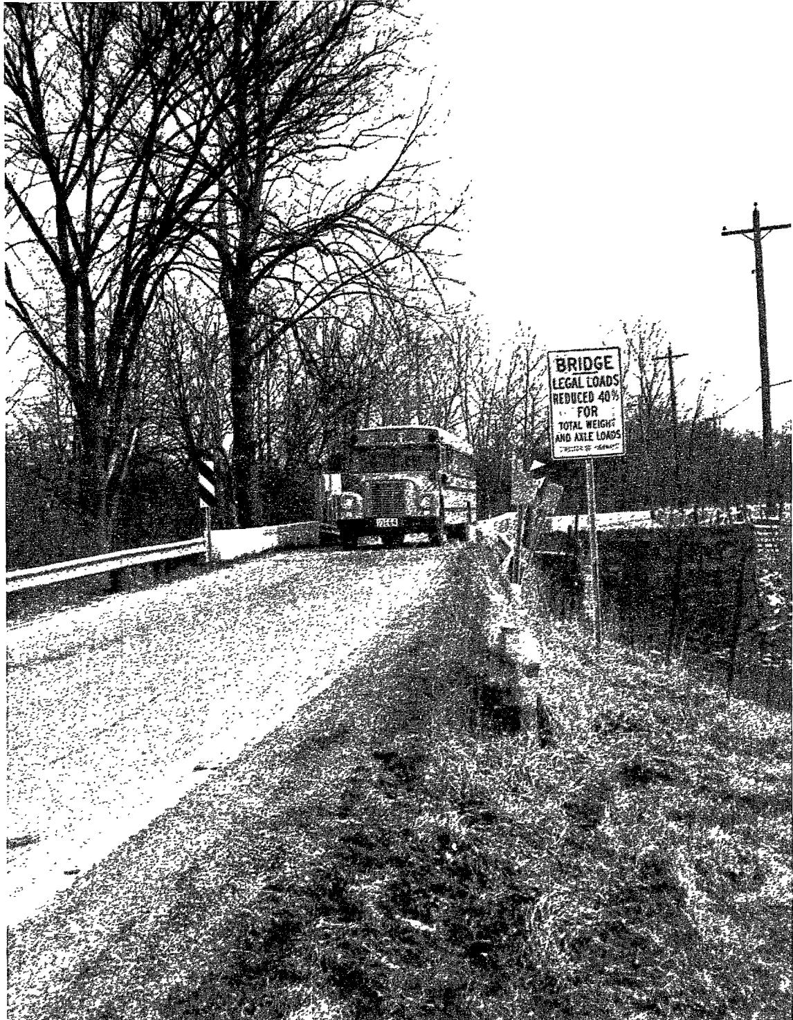
Posted bridge on Federal-aid system Route 129 in Butler County, Ohio (GAO Photograph)
