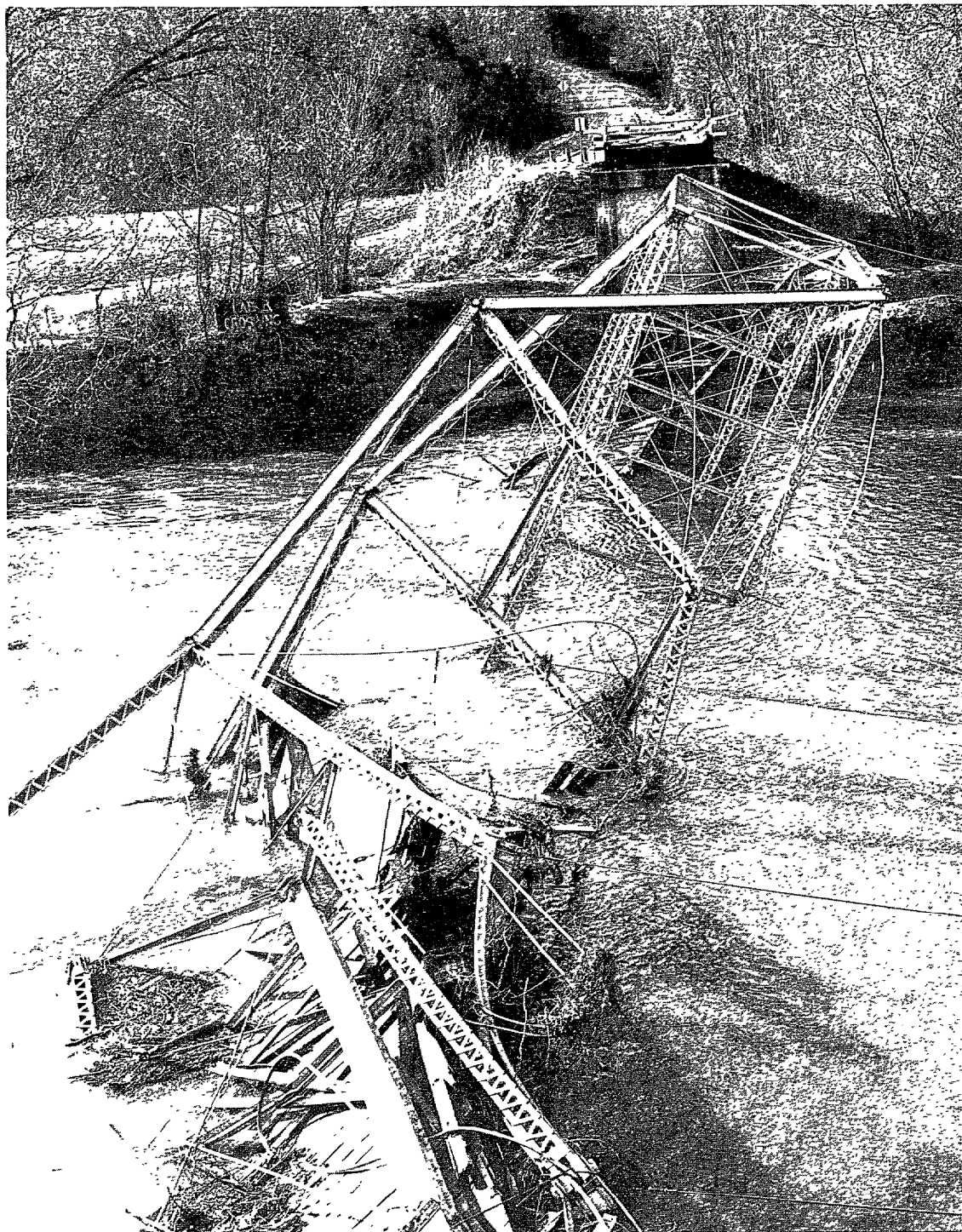
Collapsed Federal-aid system bridge on Route 1003 at the Yadkin-Serry County line, North Carolina
