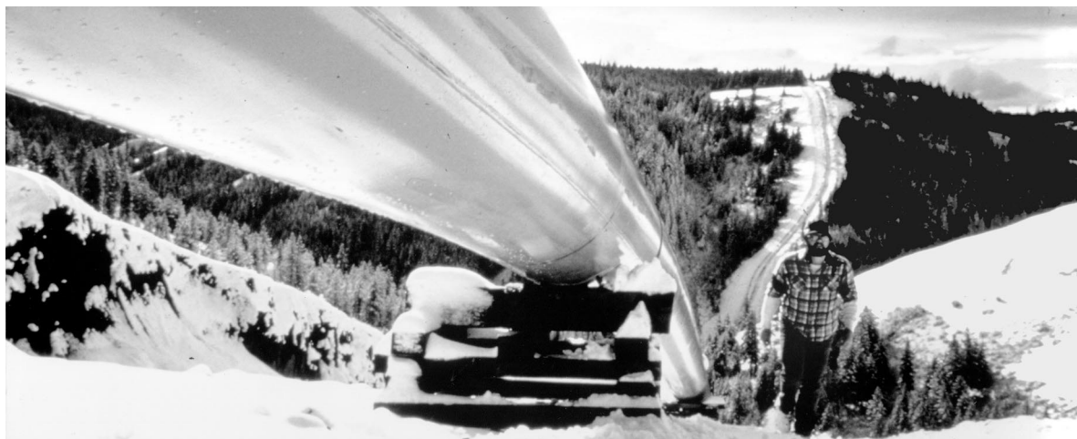
(3) An interstate system of pipelines transports natural gas to local markets in the United States. This system is composed of over 300,000 miles of piping, not including local distribution lines. Many pipelines intersect at market centers that provide numerous routes to move gas to local markets, in addition to providing related services such as short-term gas storage and gas loaning.
