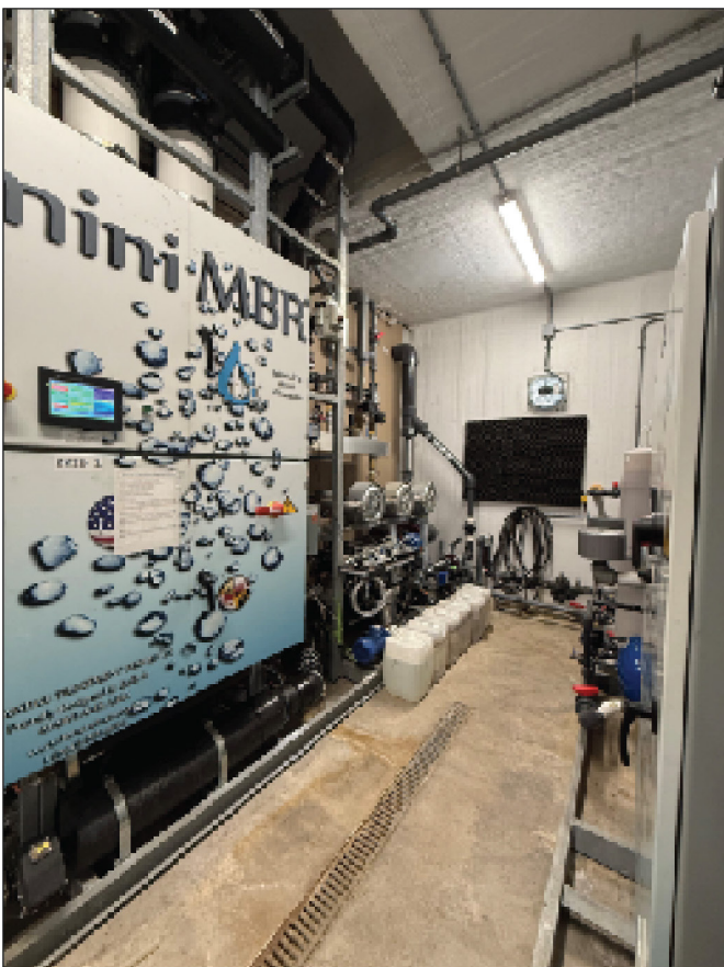
Interior of a wastewater treatment facility that serves a business park, businesses, and residences in Garrett County, Maryland.
