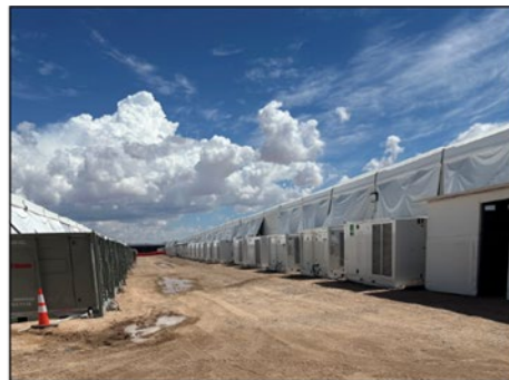
Heating, Ventilation, Air-Conditioning systems outside of Camp East Montana housing units
