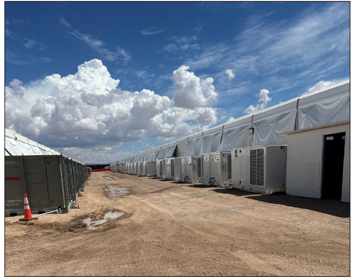
Heating, Ventilation, Air-Conditioning systems outside of Camp East Montana housing units
