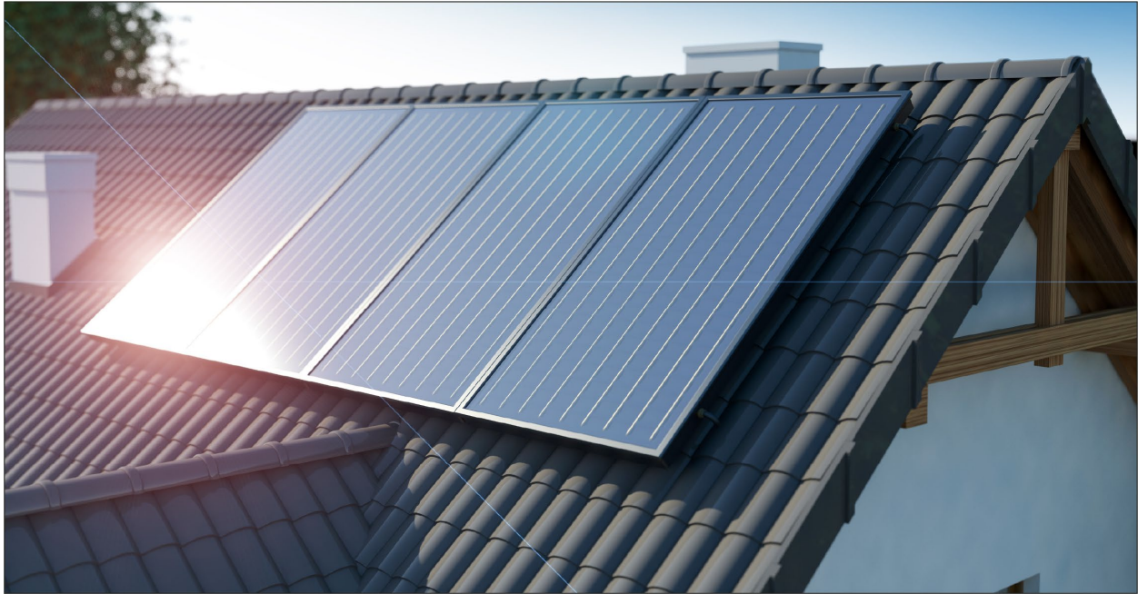
Figure 1: Residential Rooftop Solar Panels
