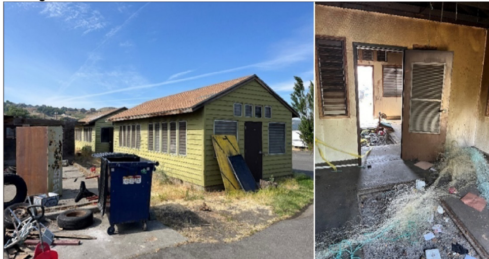
Existing fish-drying sheds, originally built in the 1970s, that the Columbia River Inter-Tribal Fish Commission (CRITFC) plans to convert into a second restroom at the site.
