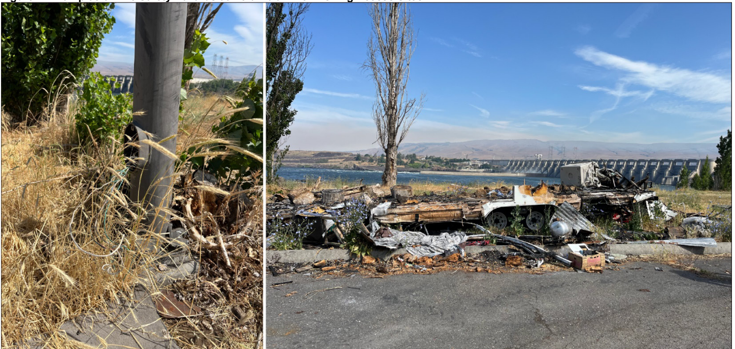
Light pole with exposed wire in tall dry grass posing risk of fire.
