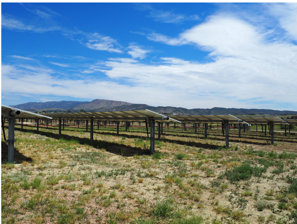
Figure 3: Example of Solar Farm Receiving Opportunity Zone Investment
