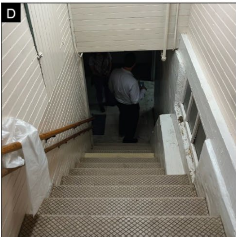
Image D: Narrow, steep stairs that provided the only access to the school cafeteria, making it difficult for teachers and children with physical disabilities to access.
