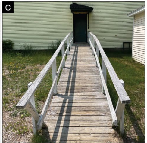
Image C: The only wheelchair accessible entrance into the school.
