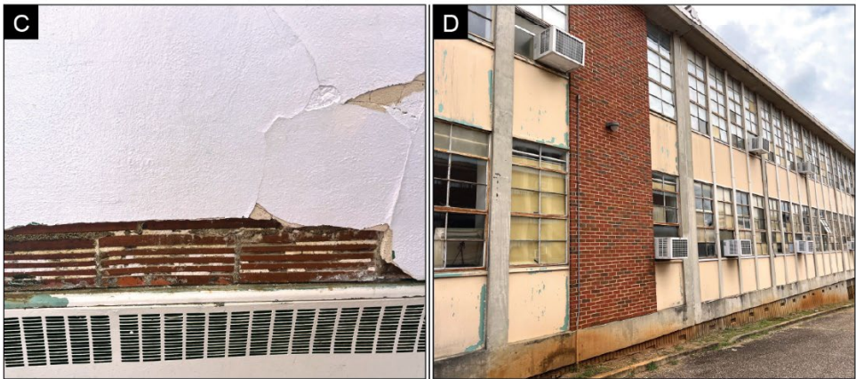
Image C: Crumbling plaster caused by excessive humidity.
