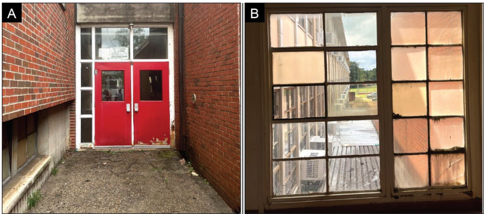
Image A: Two of nearly 100 exterior doors on the school's campus, which created security challenges.
