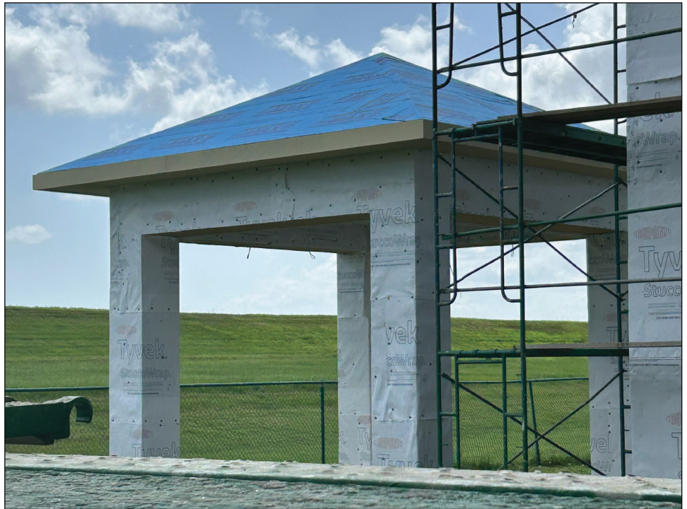
Figure 14: A Home in Louisiana with a Sealed Roof Deck—A Required Feature for Roofs Built to the FORTIFIED Construction Standard
