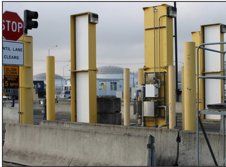
Figure 9: U.S. Customs and Border Protection’s Radiation Portal Monitor in Puerto Rico
