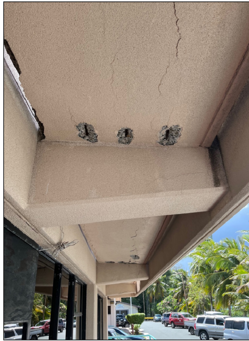
Visible water damage, exposed and rusted rebar, and cracks at Palau hospital.
