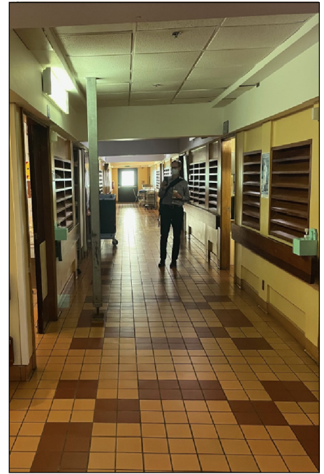
Ceiling supported by pole in hospital corridor.
