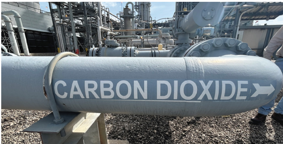
Source: GAO team photo taken with permission of Petra Nova Parish Holdings. | GAO-26-107711
