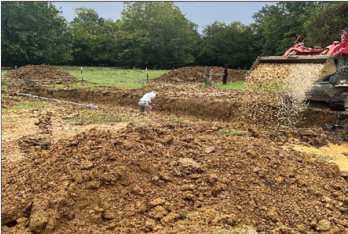
A nonprofit organization installing a new septic system for a home with inadequate wastewater treatment.
