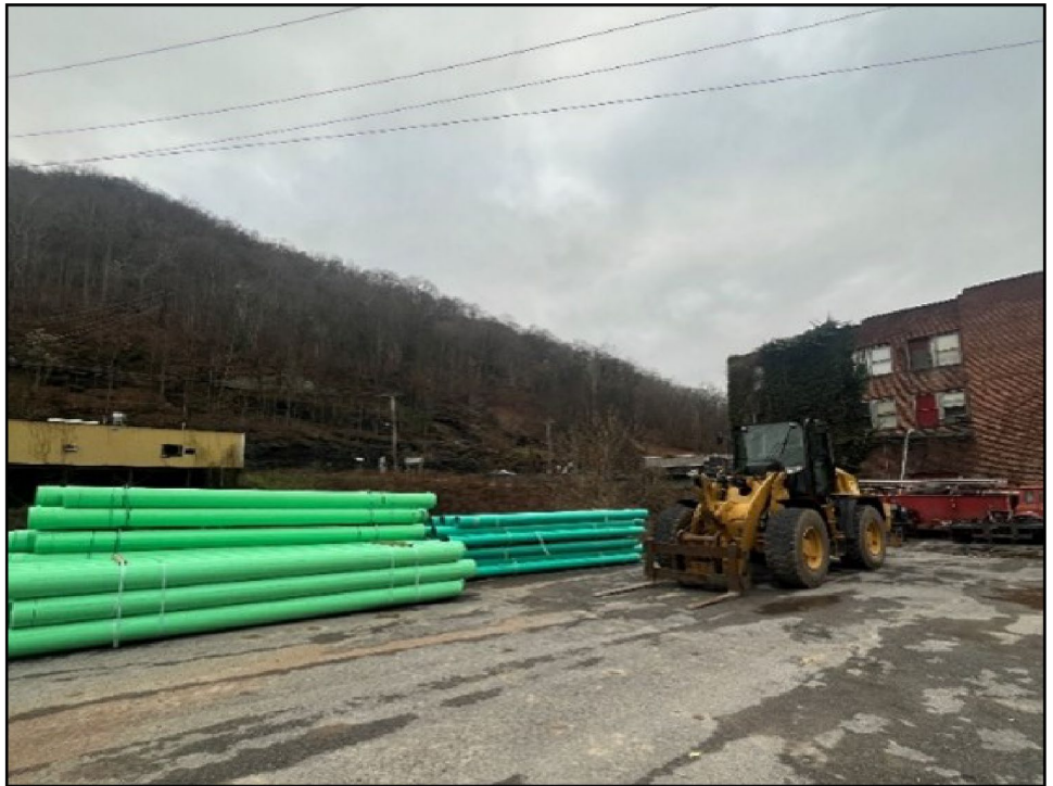
Figure 5: Construction of a Sewer to Bring Wastewater Treatment to a Rural Unserved Community in West Virginia
