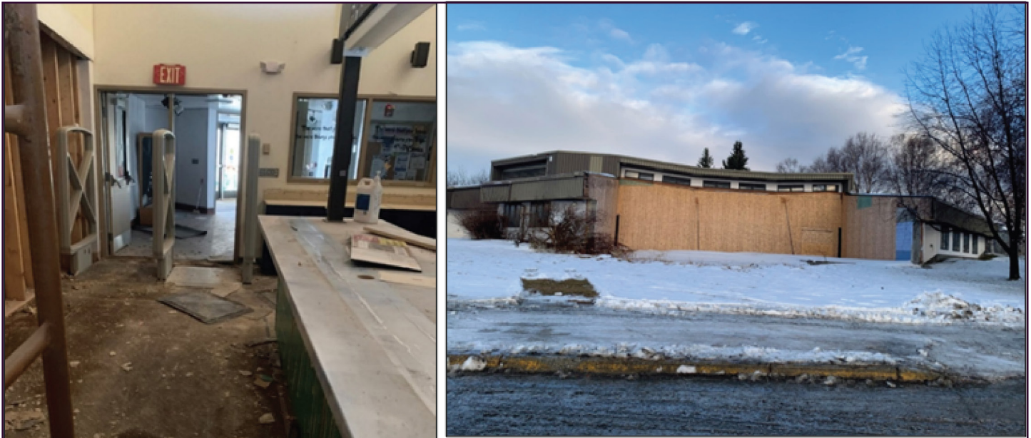
Left: Damage related to roof collapse in the lobby. Right: Boarded up exterior near area of roof collapse.
