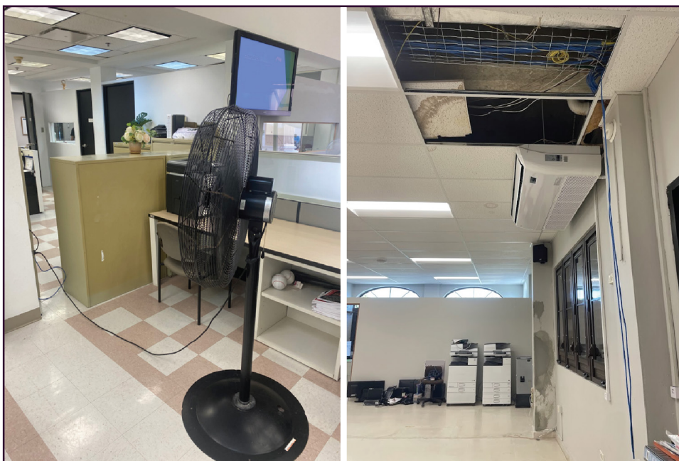
Left: In the municipal offices of a partially operational library, fans arrived after months without air conditioning. Right: In another library, three new air conditioning units were damaged after a large-scale power outage.
