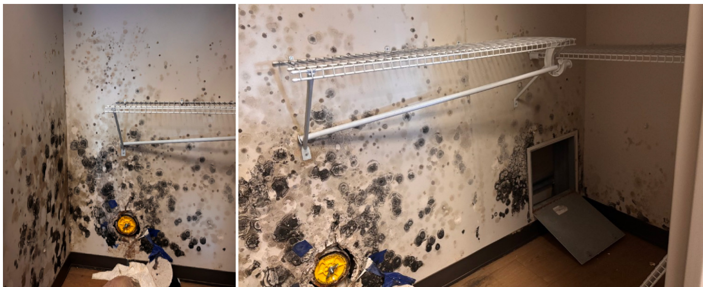
Figure 7: Suspected Mold in Barracks at Naval Station Norfolk, VA
