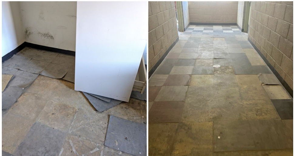
Figure 14: Barracks Water Damage and Mold Growth Caused by Flash Flooding at Twentynine Palms, October 2024
