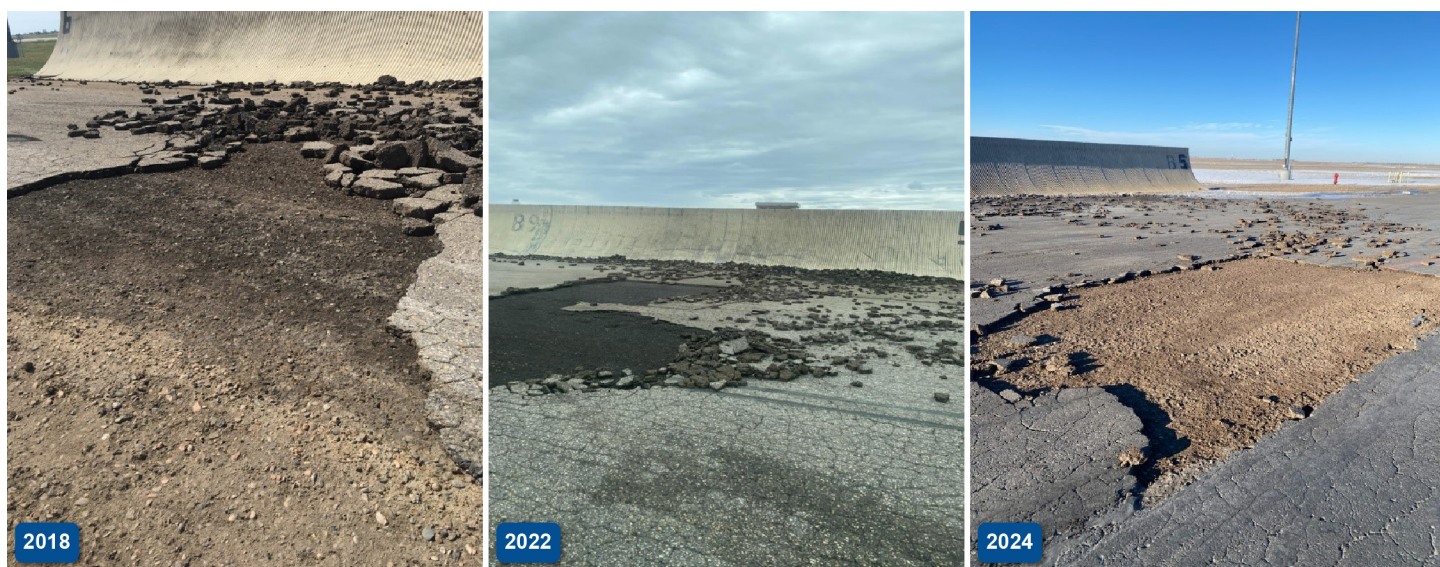
Figure 5: Damage to B-52 Parking Area at Minot Air Force Base Requiring Repairs in 2018, 2022, and 2024
