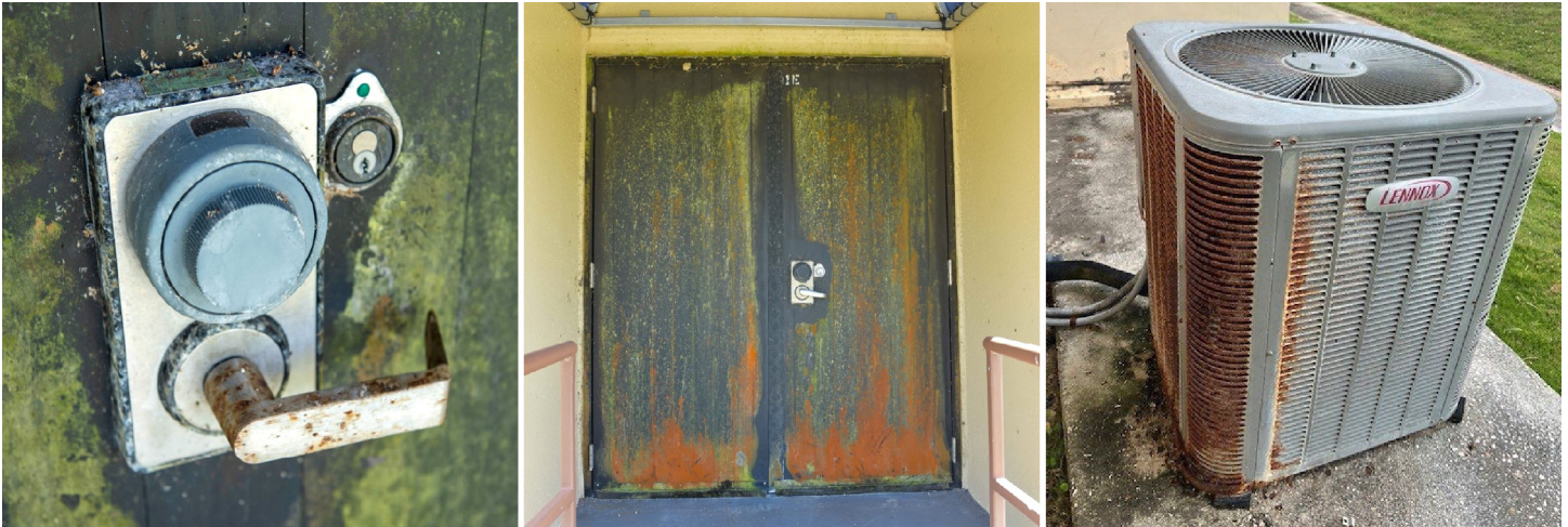
Figure 15: Corrosion and Algae on Facility Components at Naval Base Guam and Andersen Air Force Base Due to Island Climate, April 2025
