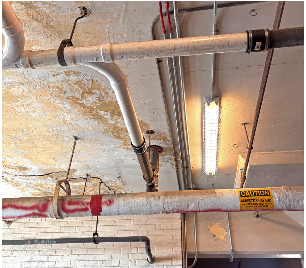
Figure 11: Water Damage and Asbestos Hazard at Aging Facility in Naval Station Norfolk, January 2025
