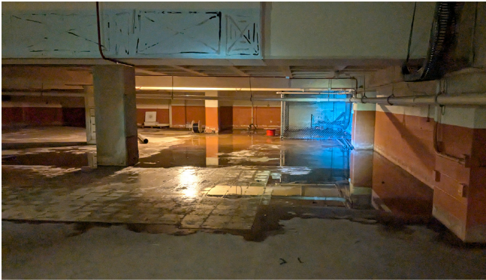
Figure 12: Water Present in Foundation of 1960s-era Building at Minot Air Force Base, September 2024
