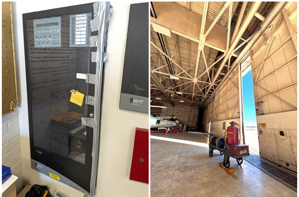
Figure 9: Barracks and Hangar with Inoperable Fire Safety Systems at Naval Station Norfolk, January 2025
