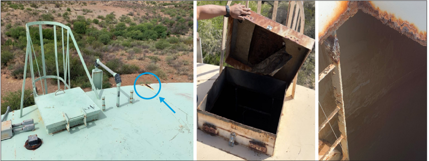
5-inch rust hole in the roof of a tank
