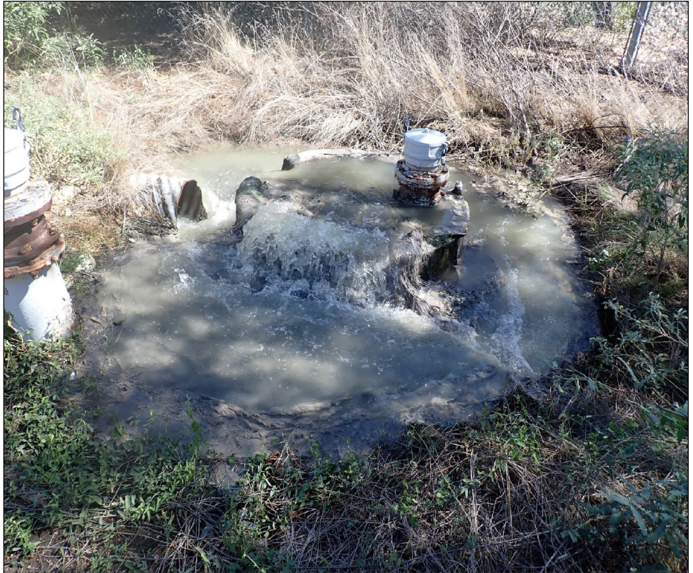
Figure 4: Lift Station Failure Resulting in Sewage Overflows
