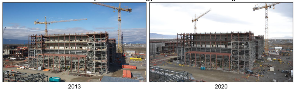
Figure: Status of Construction on the Pretreatment Facility, Part of the Waste Treatment and Immobilization Plant at the Department of Energy's Hanford Site in Washington State
