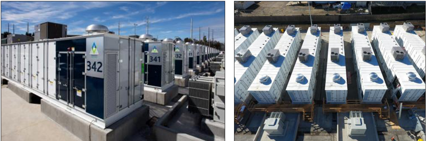
Figure 7: San Diego Gas & Electric's 30 Megawatt Escondido Energy Storage Facility
