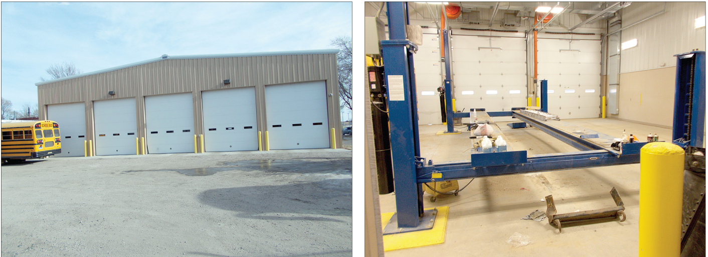
Figure 7: Exterior and Interior of Recently-Constructed School Bus Maintenance Building Where Door Does Not Close When a Large School Bus Is On Hydraulic Lift
