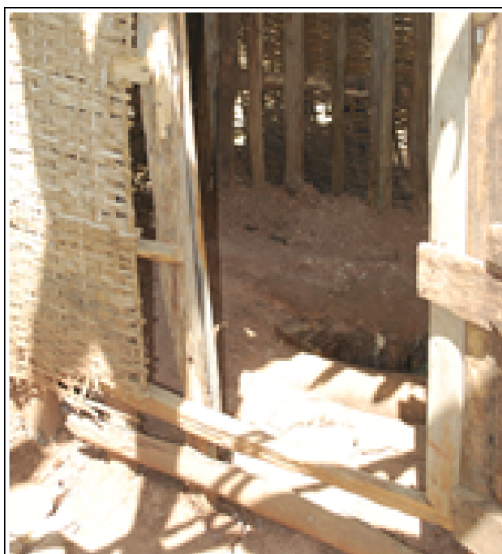
Figure 7: Basic Household Latrine Built for a USAID Water Supply, Sanitation, and Hygiene Activity in Ethiopia
