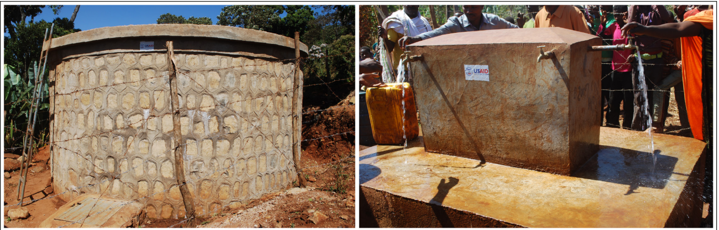
Figure 9: Drinking Water Tank and Taps Constructed as Part of USAID's WASH Activity in Buda Megada Village, Bule Hora District, Oromiya, Ethiopia
