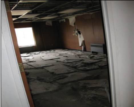
Old firehouse with collapsed ceilings.
