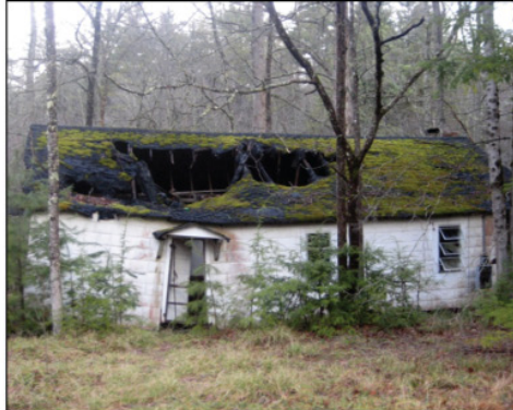
Cabin with collapsed roof.
