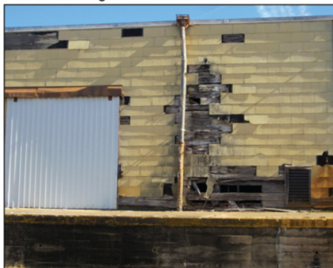
Warehouse with exterior damage.
