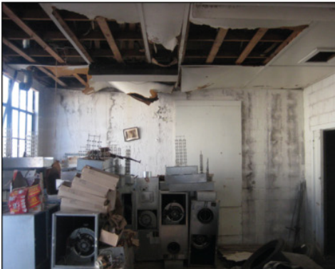
Warehouse with a collapsing ceiling.
