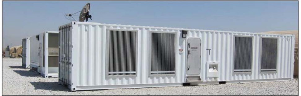
Figure 7: 1-megawatt Microgrid at Bagram Airfield
