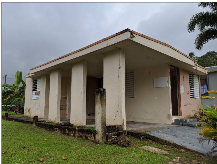
Figure 11: Damaged Public Housing units, February 2020.
