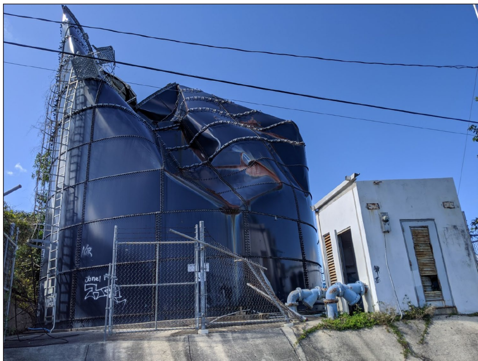
Figure 10: Damaged Water Tank, February 2020.
