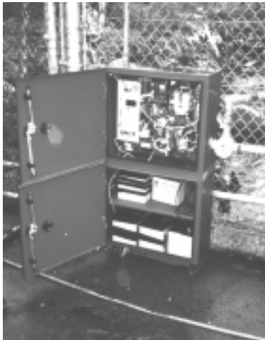
Remote Terminal Unit Controlling Motorized Gas Valve
