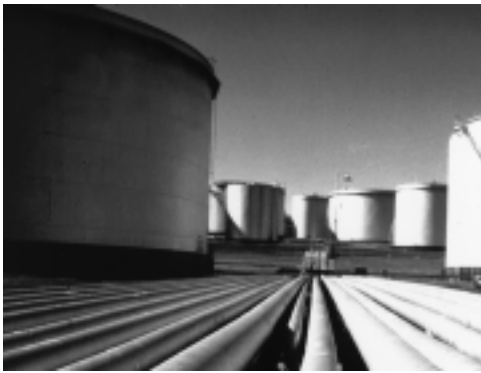
Oil Tank Farm and Pipeline Complex
