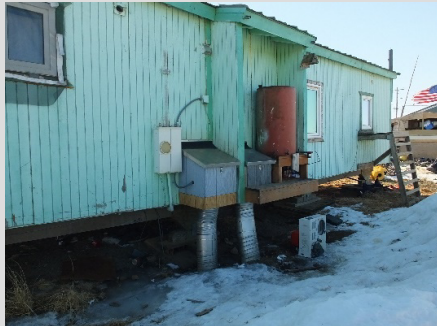
Home where newly installed pipes are separating from the home because of thawing permafrost. Pipes are inside the aluminum tubes shown under the insulated boxes.
