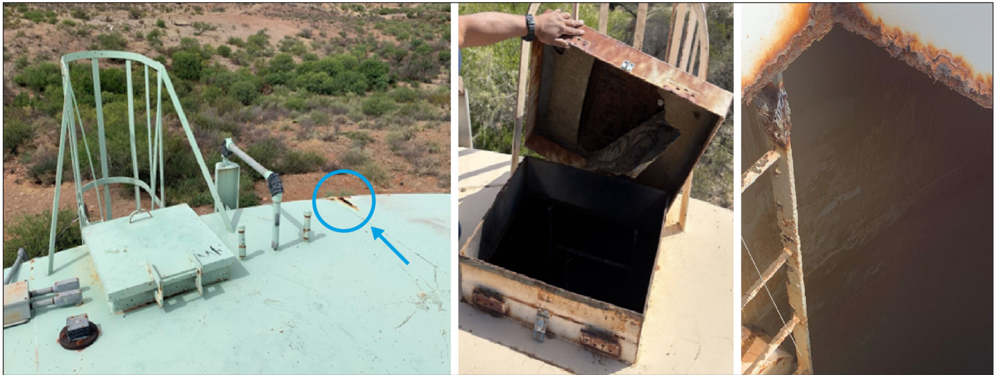
Figure 6: A Tribe's Water Storage Tanks with Severe Corrosion Because of Lack of Routine Maintenance
