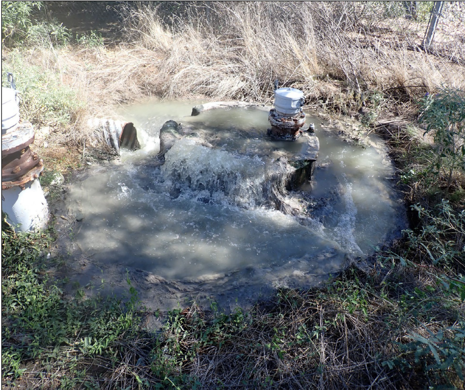
Figure 4: Lift Station Failure Resulting in Sewage Overflows
