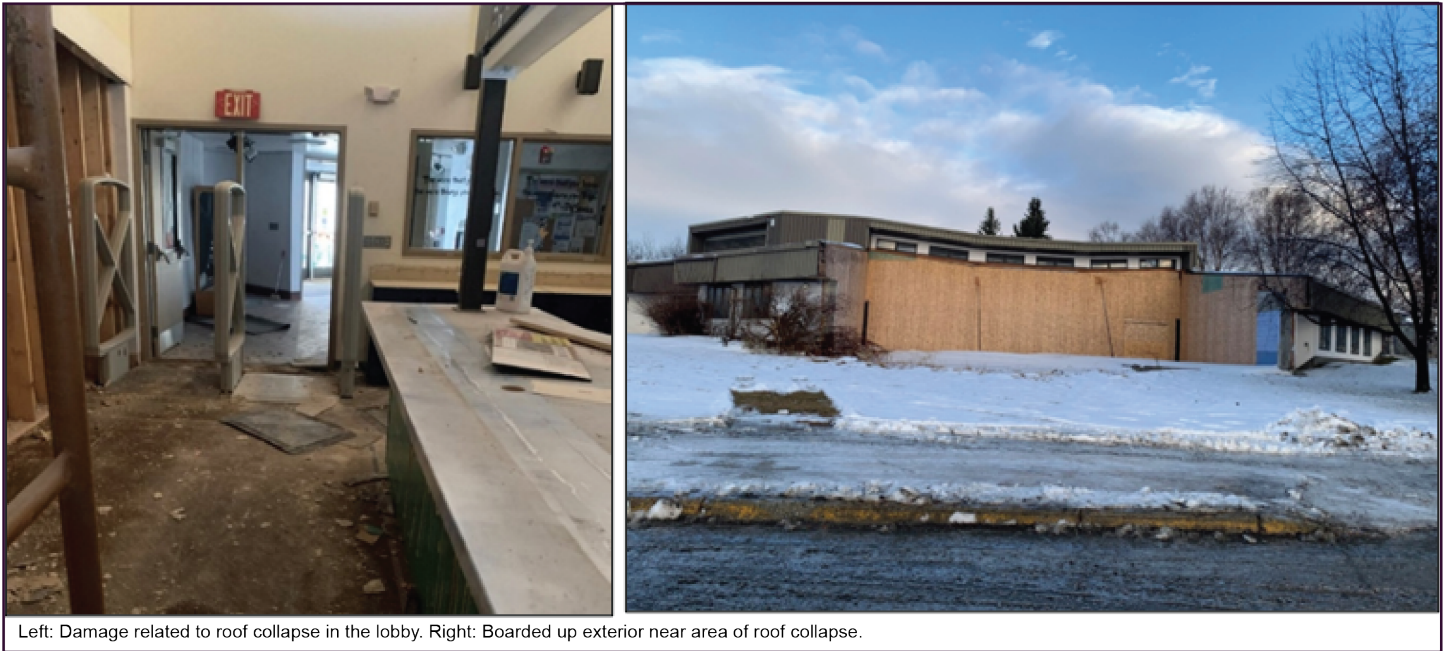
Figure 11: Interior Damage to Ceiling and Exterior of Area Related to Roof Collapse in a Now-Relocated Library in Alaska
