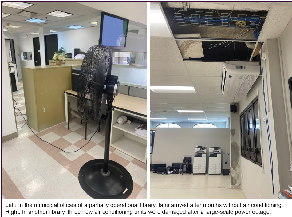
Figure 9: Two Libraries in Puerto Rico Face Malfunctioning Air Conditioning Units
