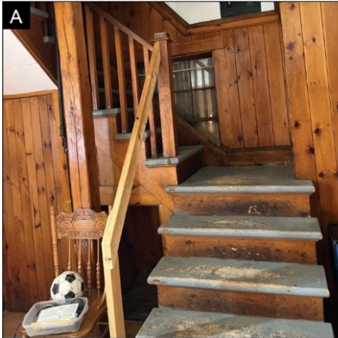
Image A: Steep stairs to access second story of a school house, making it difficult for teachers and children with physical disabilities to access.
