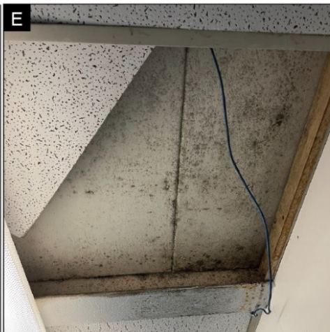
Image E: Black mold behind the ceiling tiles of the school cafeteria where the children ate lunch every day.
