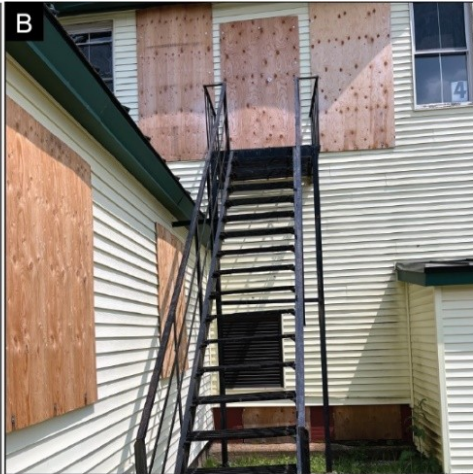
Image B: Fire escape that had gaps in the railings large enough for an elementary-aged child to fall through. The fire escape was also not secured to the ground properly and not safe to bear weight.
