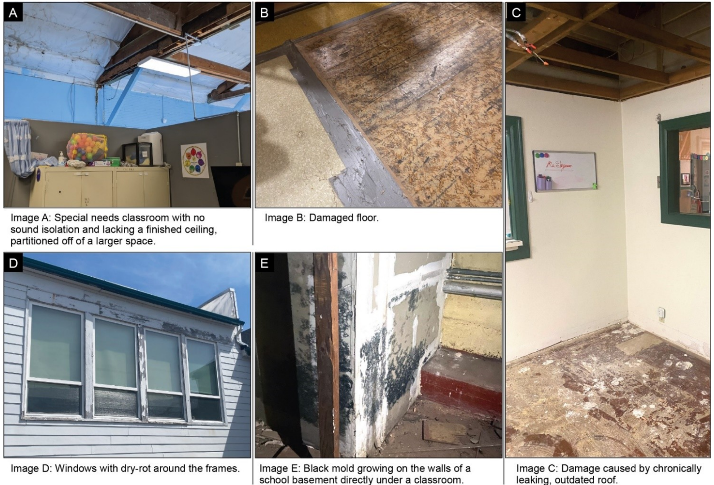
Figure 2: Photos of an Over-100-Year-Old Rural Elementary School with Significant Facility Issues, School Year 2024-25
