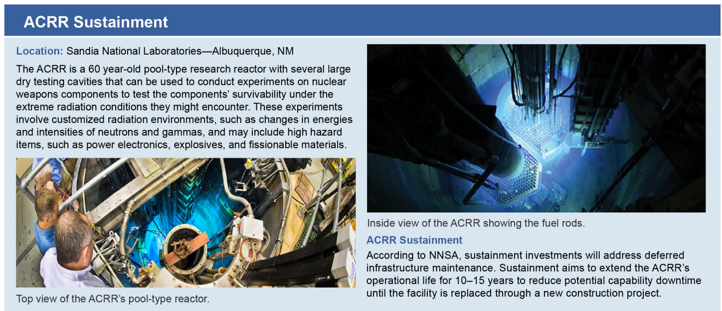
Figure 4: Annular Core Research Reactor (ACRR) Sustainment
