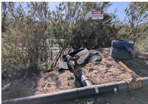
The surface water diversion system at the Moab Mill Site, which helps protect endangered fish species in the Colorado River.
