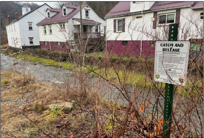
Homes discharging untreated wastewater directly into a stream, creating health risks and limiting fishing.
