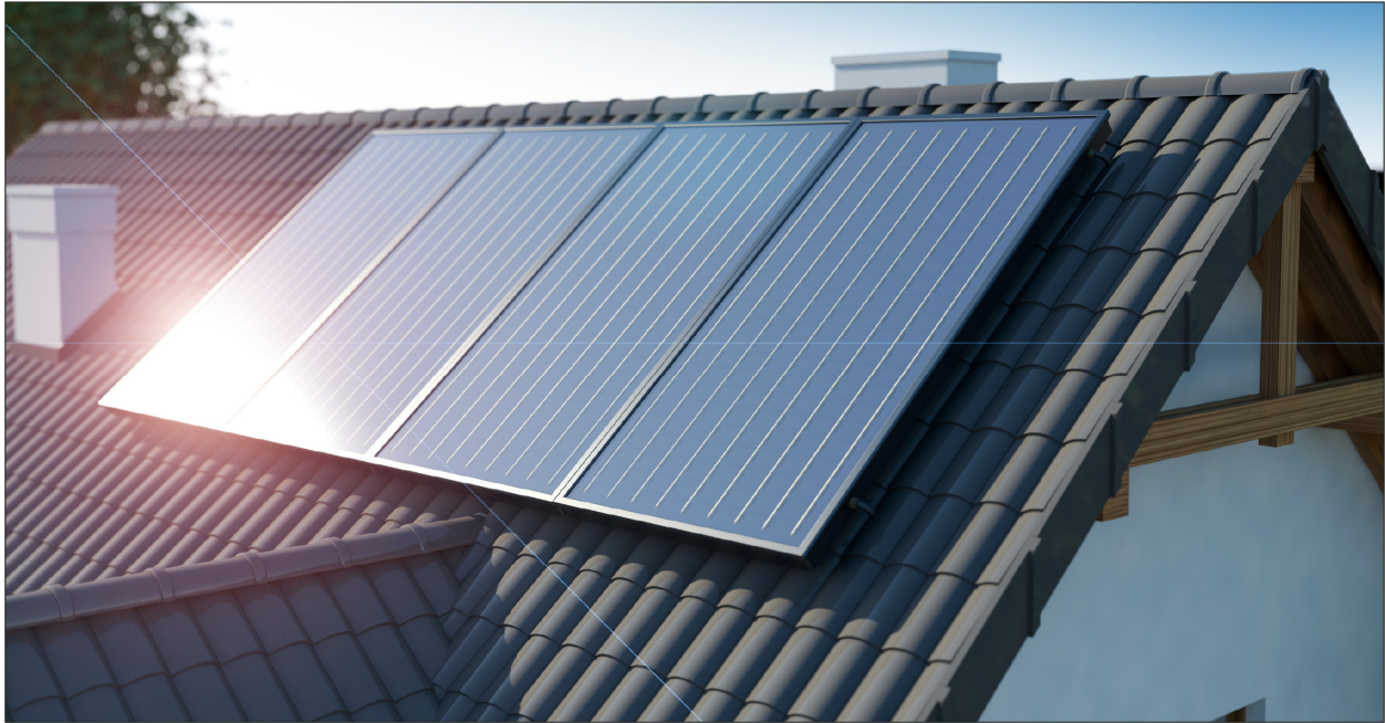
Figure 1: Residential Rooftop Solar Panels
