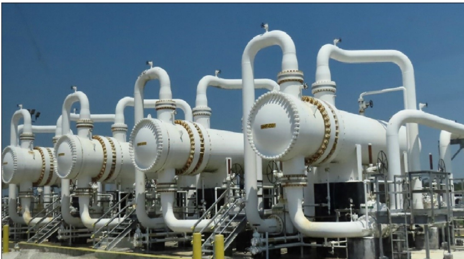
Figure 8: Heat Exchangers at the Big Hill Strategic Petroleum Reserve Site
