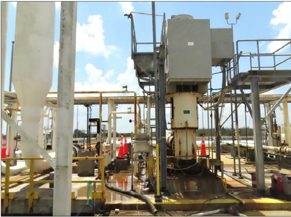
Figure 7: Leaking Brine Disposal Pumps at the Big Hill Strategic Petroleum Reserve Site
