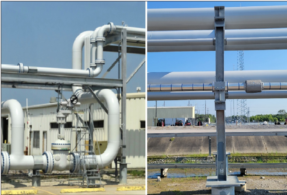
Figure 5: Life Extension Phase 2 (LE2) Project Work Quality Issues at the Bayou Choctaw Strategic Petroleum Reserve Site
