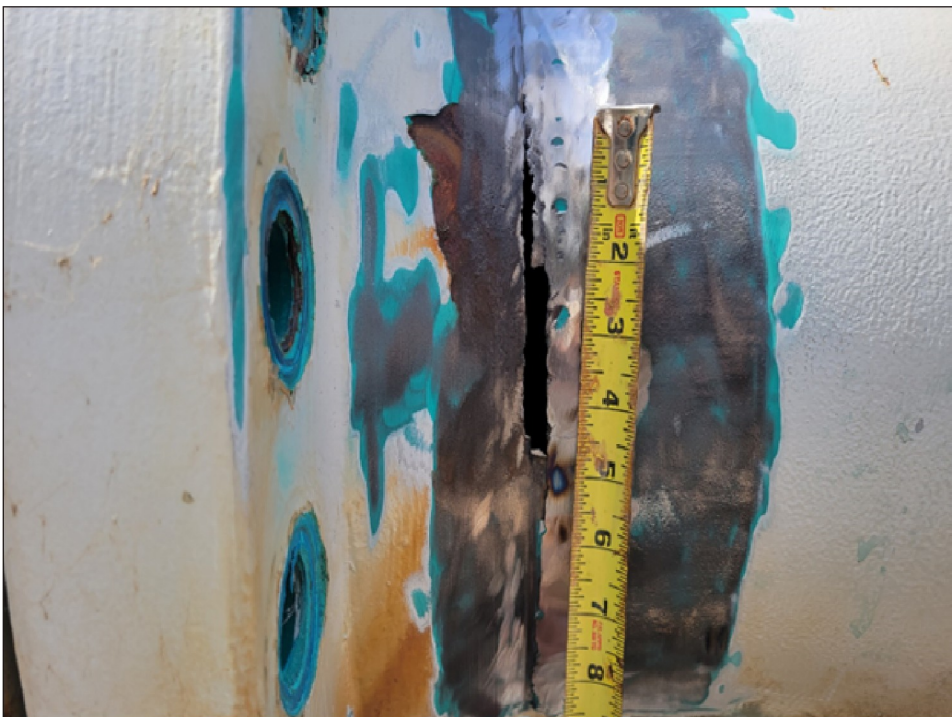
Figure 4: Leaking Raw Water Pipe Requiring Repair During 2022 Drawdown at the West Hackberry Strategic Petroleum Reserve Site
