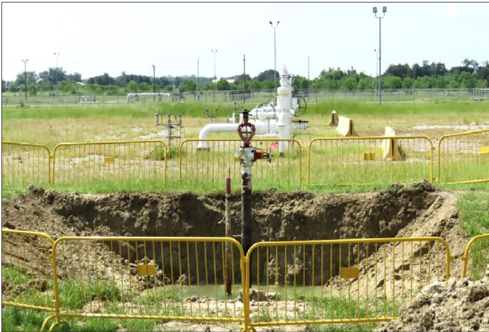
Figure 6: Leaking Fire Suppression System at the West Hackberry Strategic Petroleum Reserve Site
