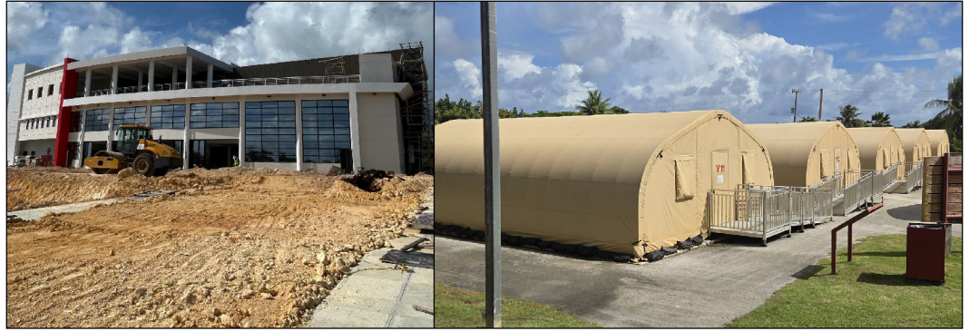
Figure 10: Northern Marianas College's Student Center Under Construction and Temporary Classrooms Built After Super Typhoon Yutu
