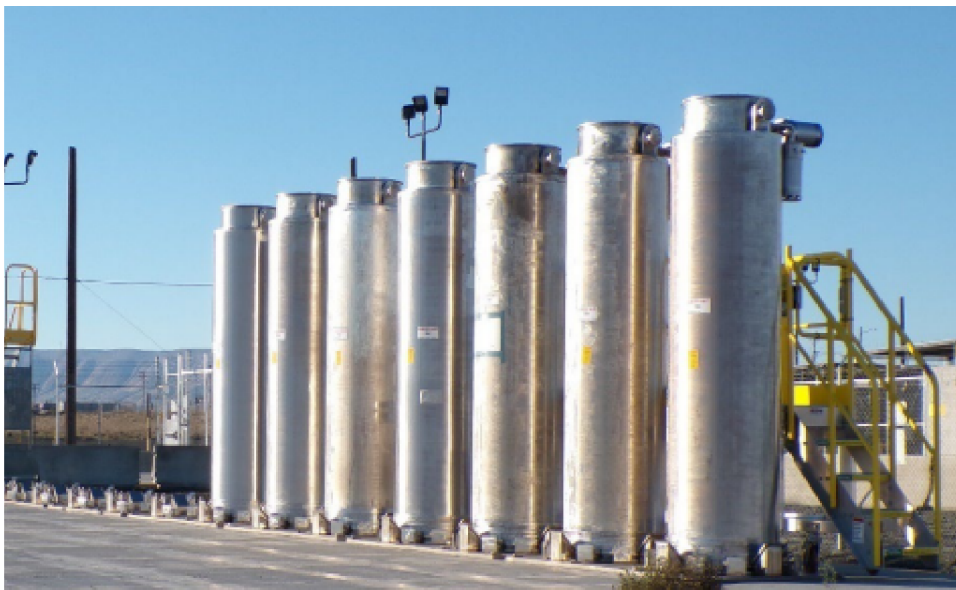
Figure 6: Ion Exchange Columns on a Storage Pad at the Department of Energy Office of Environmental Management’s Hanford Site
