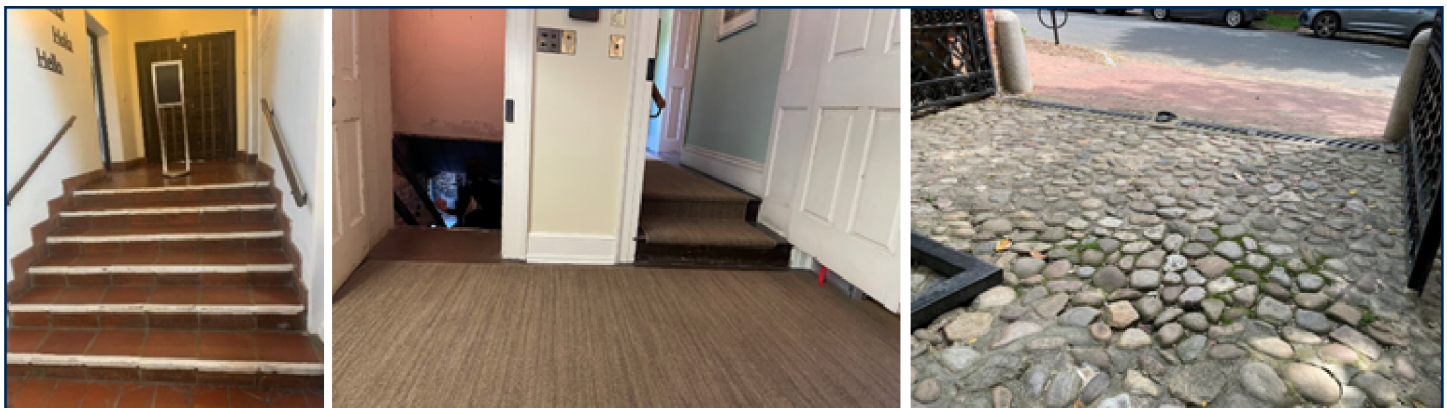
Left: Steps at the entrance of a historic site in California, with no accessible alternative. Middle: One of several steps within the first floor of one historic house in the District of Columbia. Right: Cobblestone path to enter the grounds of the same historic house.
