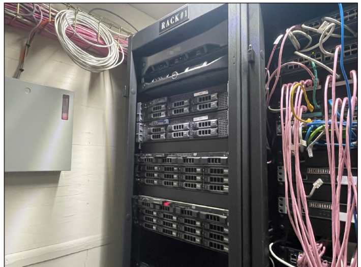
Computer system server upgrades
