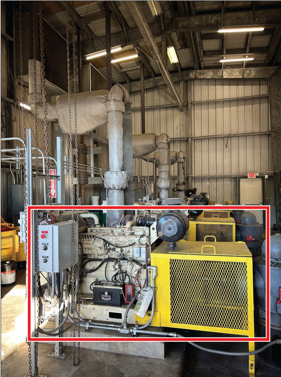
Figure 3: FEMA Hazard Mitigation Grant Program Project Using CDBG-MIT Funds for the Cost-Share Requirement: Conway Bayou Pump Station
