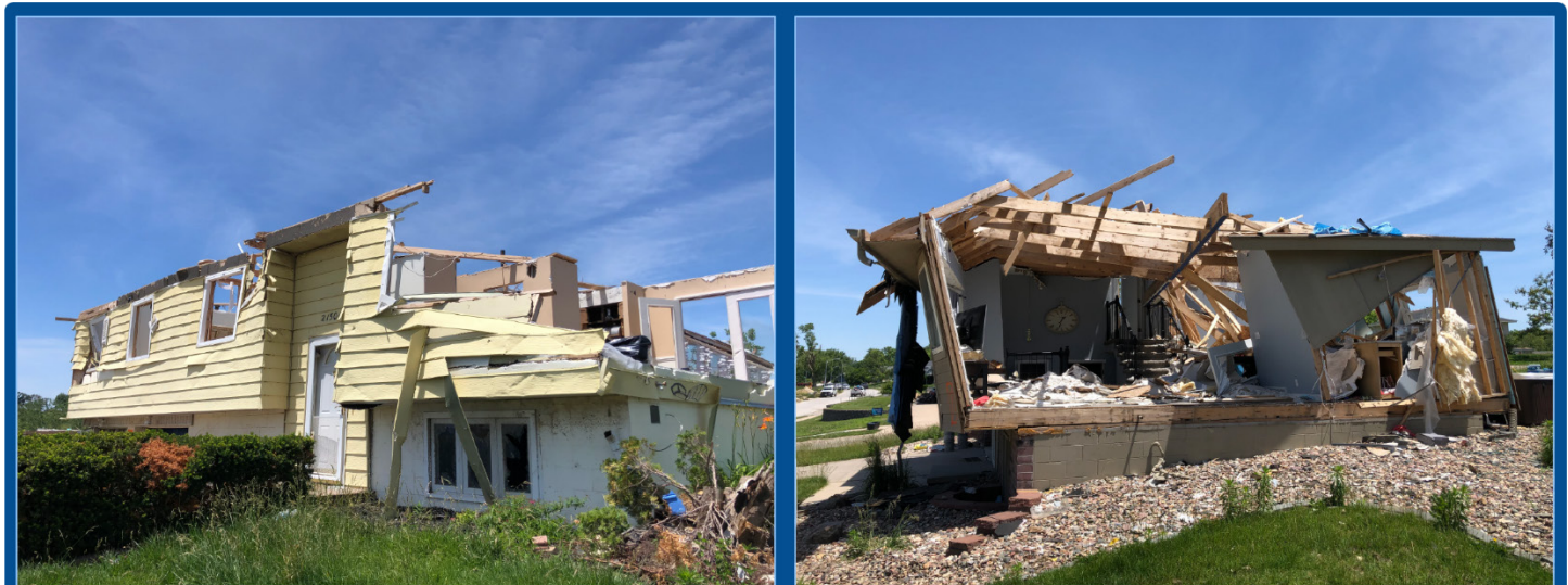
Homes in Elkhorn, Nebraska damaged in the April 2024 tornado disaster
