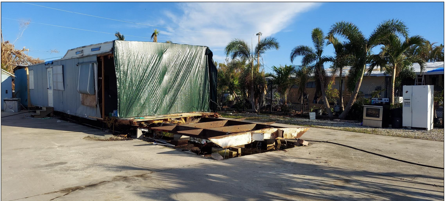
Figure 2: Hurricane Ian Damage to Home in Pine Island, Florida
