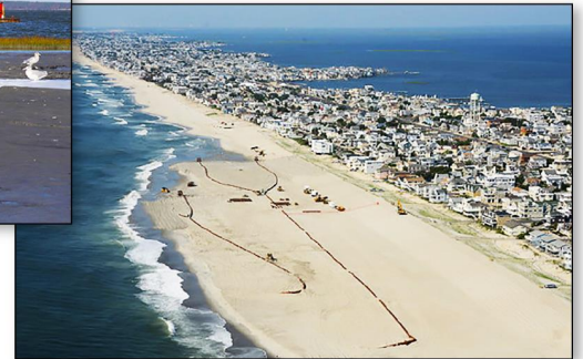
Step 3: Sand is deposited on the shore to replace sand that has been eroded or to build dunes on the beaches.
