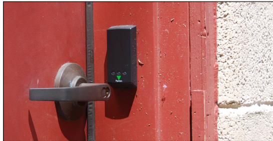
An electronic key card access installed on a facility at a Fish and Wildlife Service field unit prevents public access to administrative offices.
