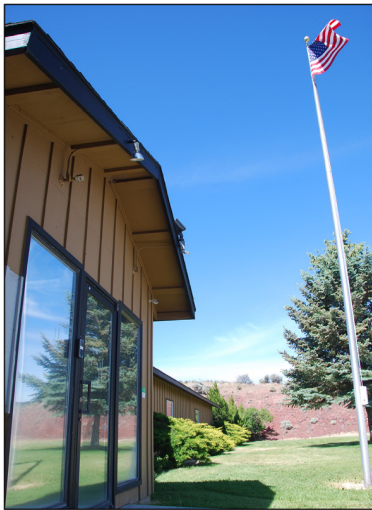
Blast-resistant film reflects the exterior landscape at a Bureau of Land Management field unit.
