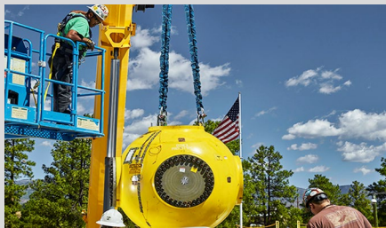
Steel vessel at Los Alamos's DARHT facility.
