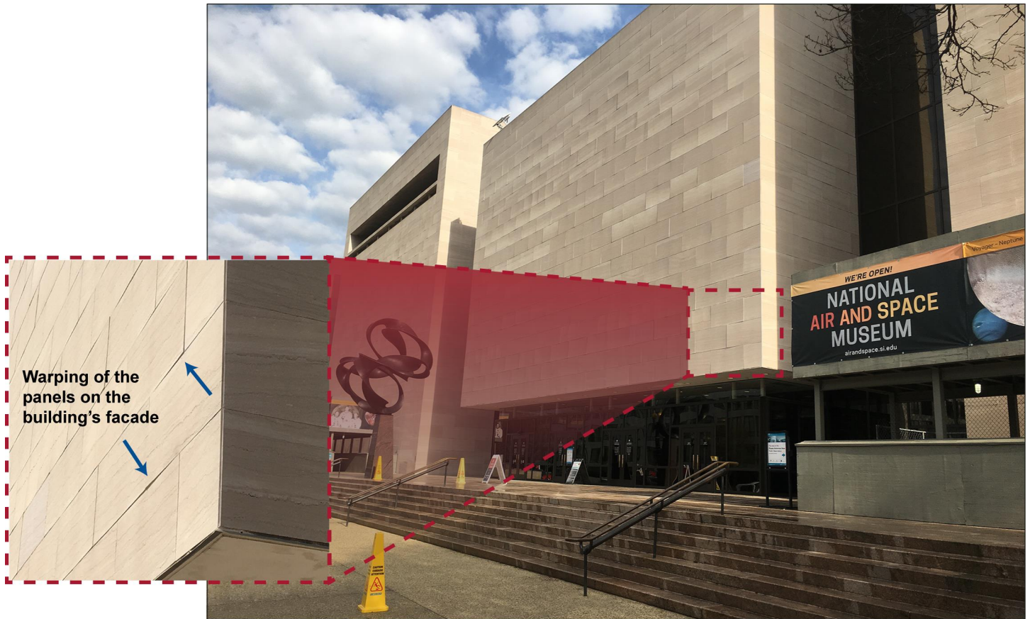
Figure 2: Warping of the Exterior's Limestone Panels at the Smithsonian's Air and Space Museum
