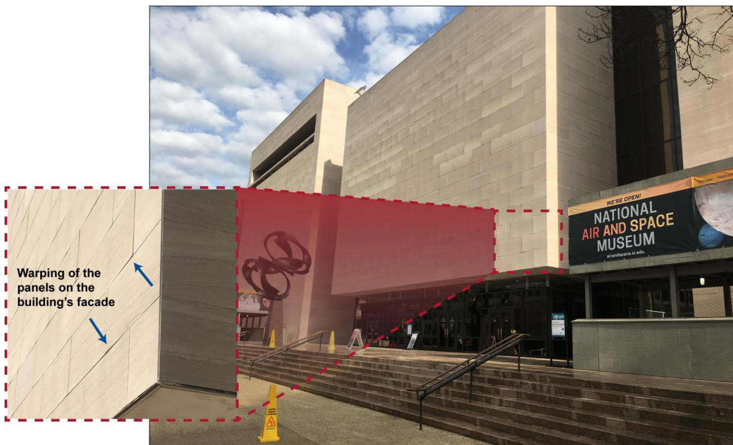
Figure 2: Warping of the Exterior's Limestone Panels at the Smithsonian's Air and Space Museum
