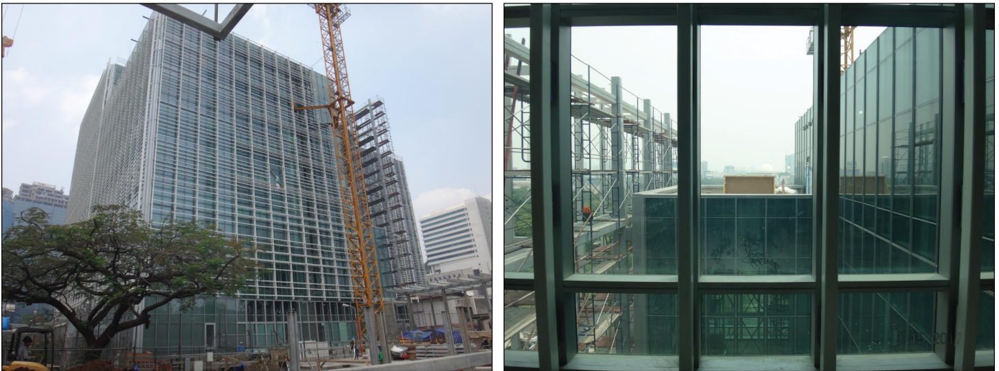
Figure 10: Exterior and Interior Views of U.S. Embassy Jakarta’s Glass Curtain Wall, under Construction during GAO Site Visit in September 2017
