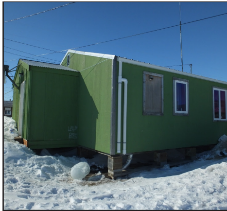
Rainwater catchment pipes on side of home.
