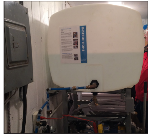
In-home storage tank for treating rainwater.
