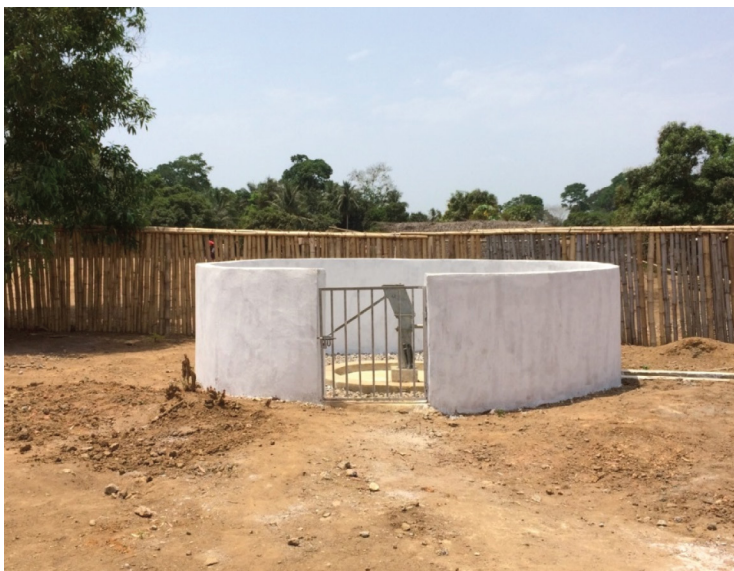
Figure 9: Water Well at a Maternal and Child Health Post in Sierra Leone Installed by a USAID Ebola Recovery Project
