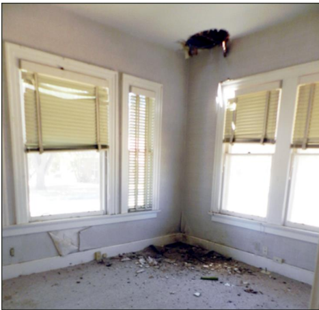
Interior damage of Kerrville Medical Center.
