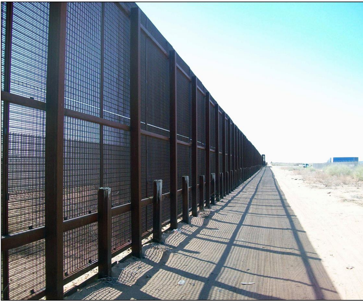
Modern double steel mesh style pedestrian fence
