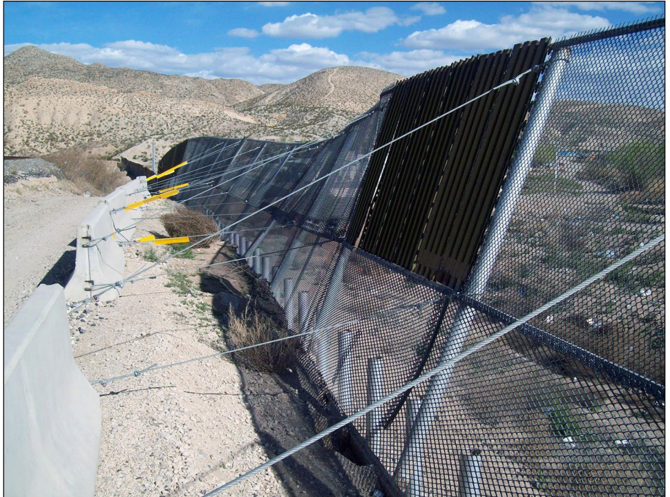
Figure 9: Legacy Pedestrian Fencing in Sunland Park, New Mexico, March 2016
