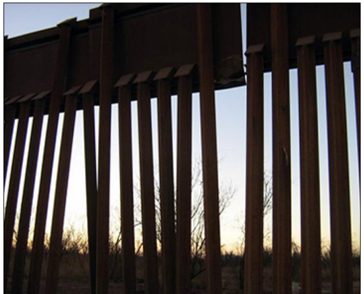
Breach in modern bollard pedestrian fencing
